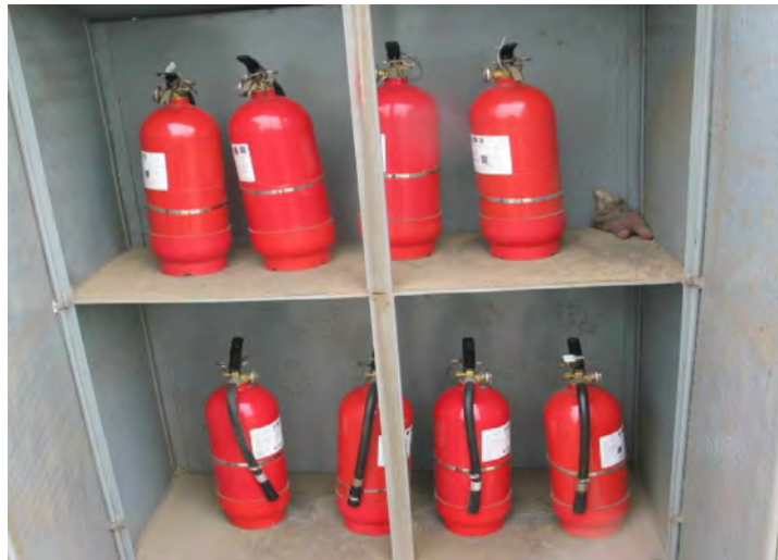
Fig. Annex- 35 Examples of materials for extinguishing fire in the landfill area
